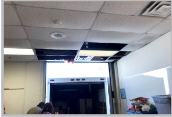
Sprinkler Line Issues
