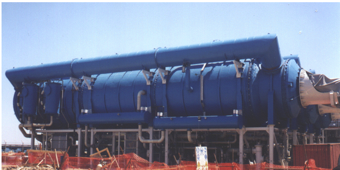
Figure 4: 8 x MVC 3,000 operating since 1998/9 in two Refineries
