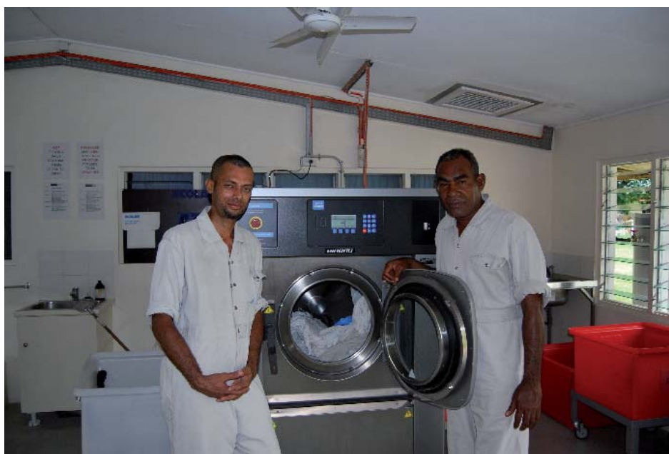
New laundry machine for West
