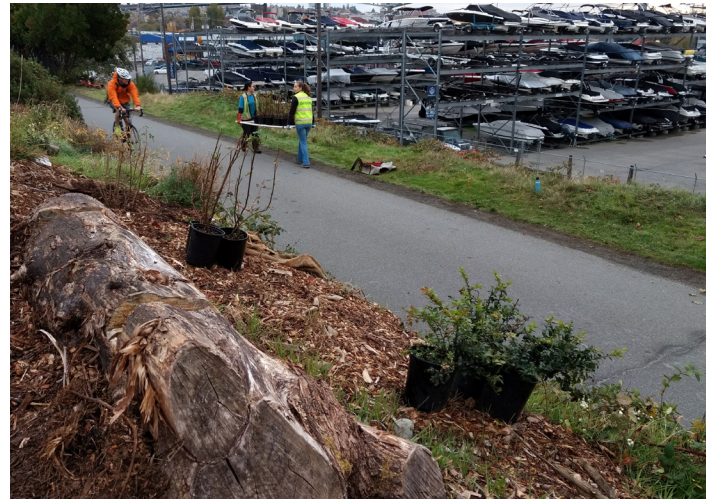
Figure 7. Woody debris installation and plants staged in 'species clumps' on the Burke Gilman trail, Seattle, WA. Photo: Matthew B Schwartz
