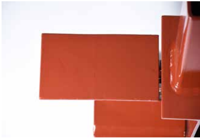
▲ AESS 3: Joint gap tolerances minimized, butt and plug welds ground smooth and filled.
