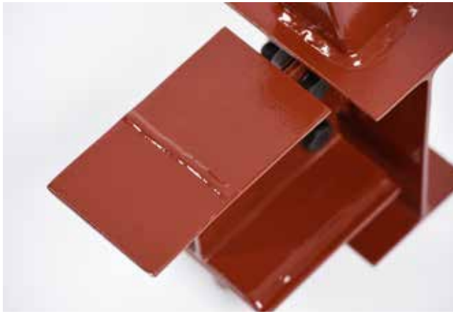
▲ AESS 2: Standard joint gap tolerances.
