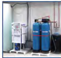
Pro Ice Reverse Osmosis Water Treatment
