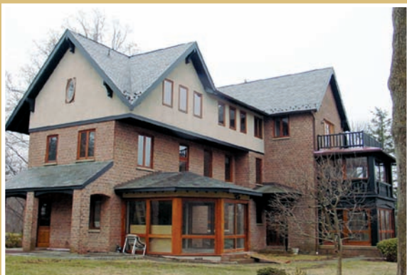
Ten-year-old slate roof on a private residence condemned by roofing contractors. The nominal snow guard damage, however, was covered by homeowner's insurance; the roof did not need to be replaced at all. (Photo by Joseph Jenkins.)
