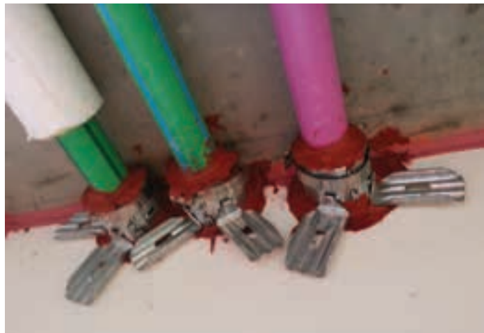
Special Inspectors will be able to assist and detect the differences between proper and improper firestop installation.
