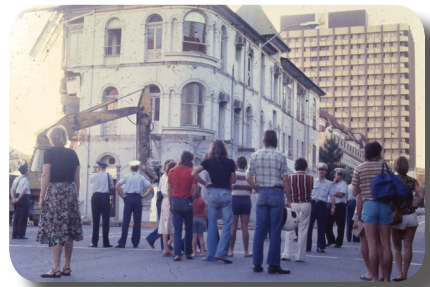
Crowds held back by Qld police during the demolition of the Bellevue Hotel in George St. on 20 April, 1979. Photo: R. Gwyther
