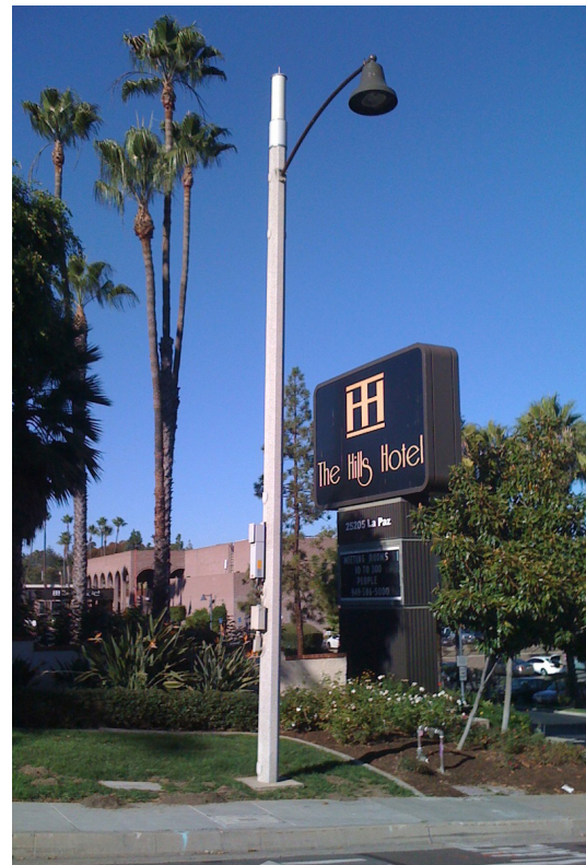
Figure 4: Omni-Directional antenna, Courtesy of Crown Castle
