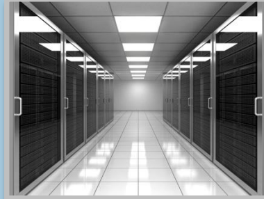
Data Center Consolidation
