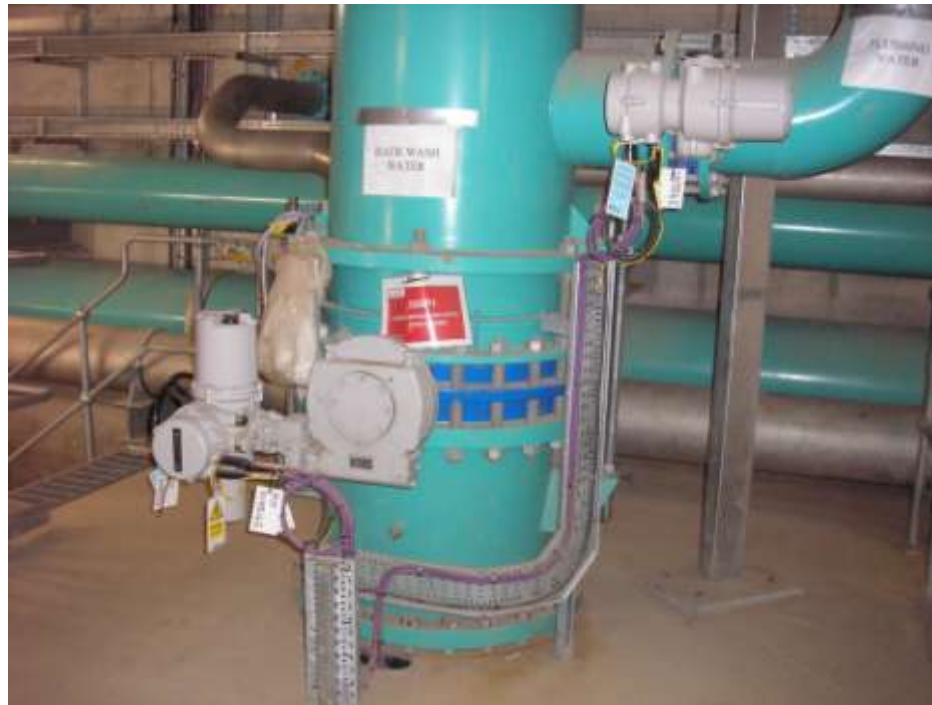
Actuators networked using Profibus
