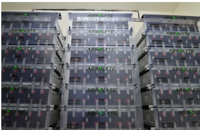
Top: Canyonlands Research Center / Dugout Ranch entrance. Middle: Evaporative cooler anchored to the lab wall. Bottom: New solar battery bank. Photos by Philip Adams
