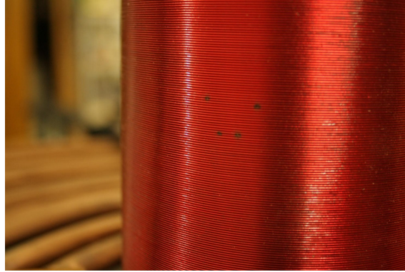
Figure 4.29: Results of inadequate space between the coils : arcing between the two occurred, burning the secondary coil at several points.
