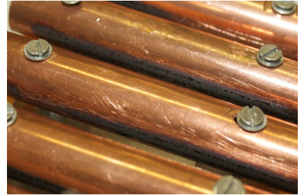
Figure 4.24: Heavy corrosion between the copper tubes.
