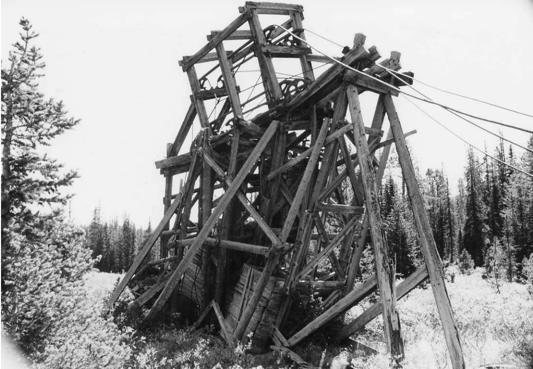
Figure 4-32. A partially collapsed counterweight tower (1990 GCM file photo).
