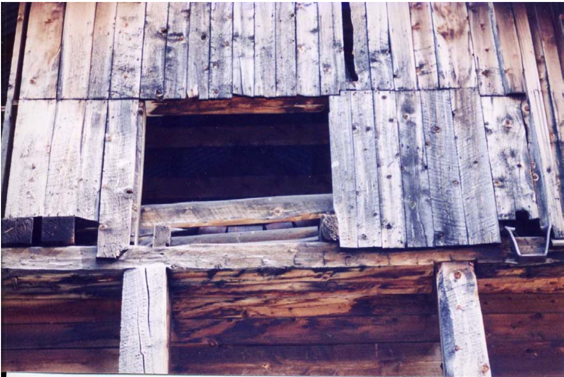
Figure 4-39. Conveyor belt rollers are visible in the upper level of the Gold Dust ore bin.
