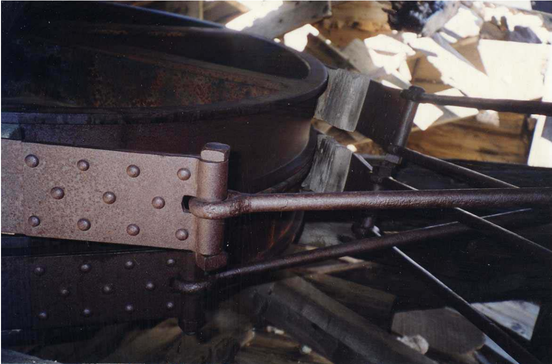
Figure 4-17. Detail of the friction brake system at the upper terminal, located below the bull wheel.
