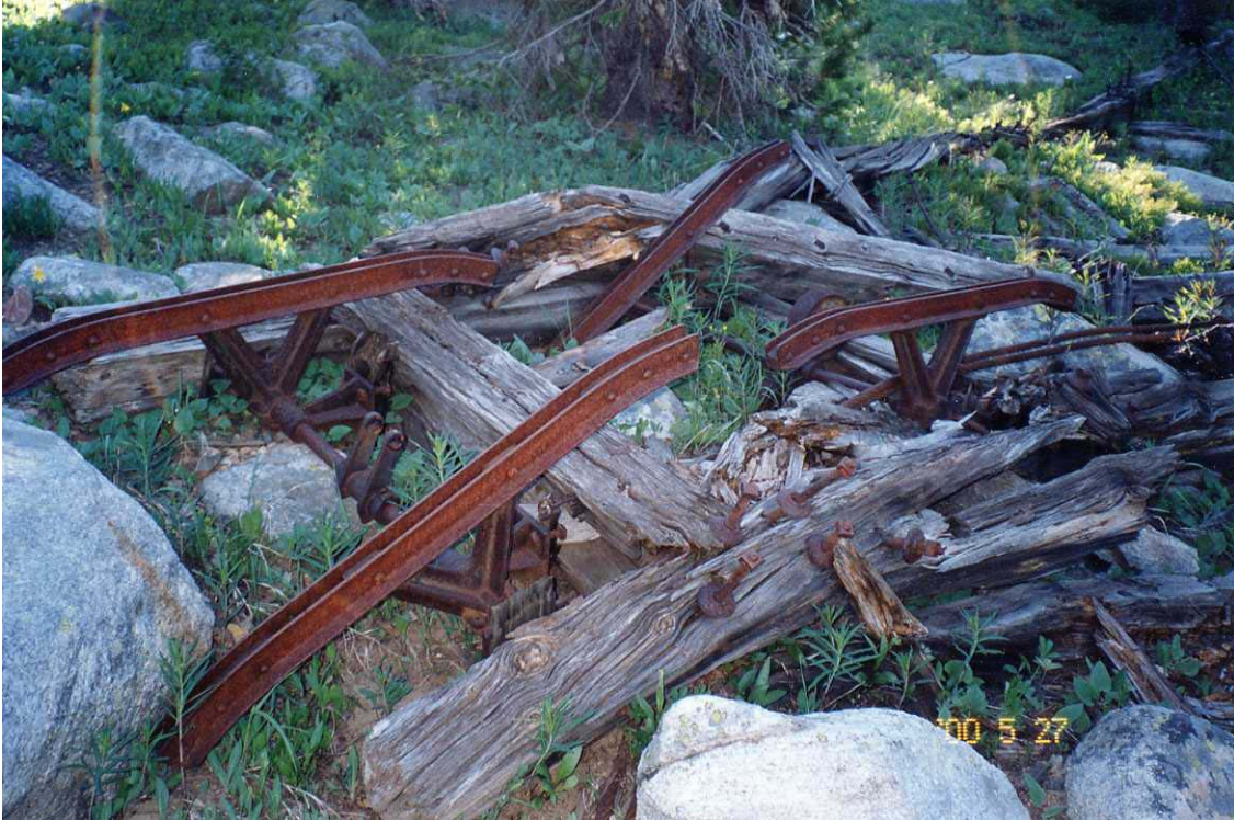
Figure 4-43. Collapsed lower tram support tower remains as they are now found.
