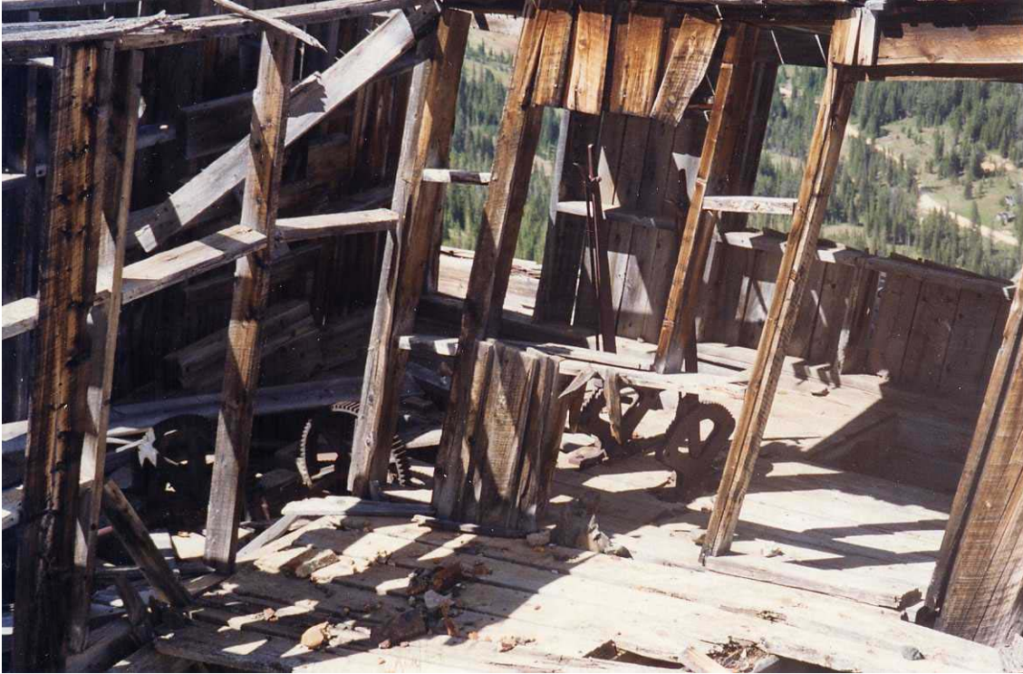
Figure 4-22. Brake house with detaching mechanism, and loading and brake controls on a ratchet system visible on the floor.
