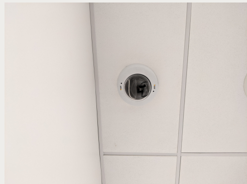
Break-Out Room Overhead Cameras
