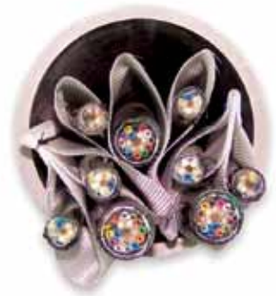
3" 3-Cell packs holding 9 cables in 4" conduit
