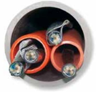
Micro MaxCell overriding existing cable plant in a 3" duct
