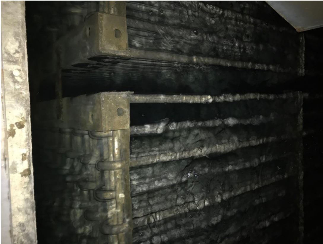
Interior View of Ice Tank Glycol Coil
