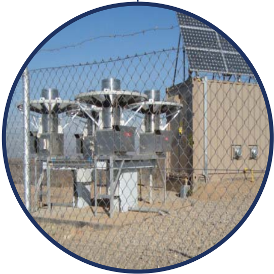
Pipeline: 2000 watt TEG and Photovoltaic - Kazakhstan Pipeline
