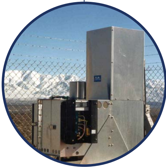
Production: 220 watts gas production and cathodic protection - Argentina
