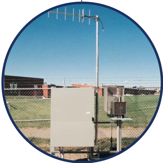
Gas Distribution: 15 watts gas pipeline distribution metering station - Calgary, Canada
