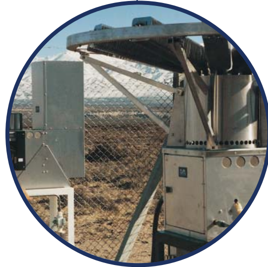
Pipeline: 220 watts and 550 watts cathodic protection and communications - Andes Mountains, Argentina
