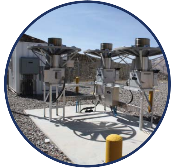
Pipeline: 1500 watts pipeline block valve station - Andes Mountains, Peru
