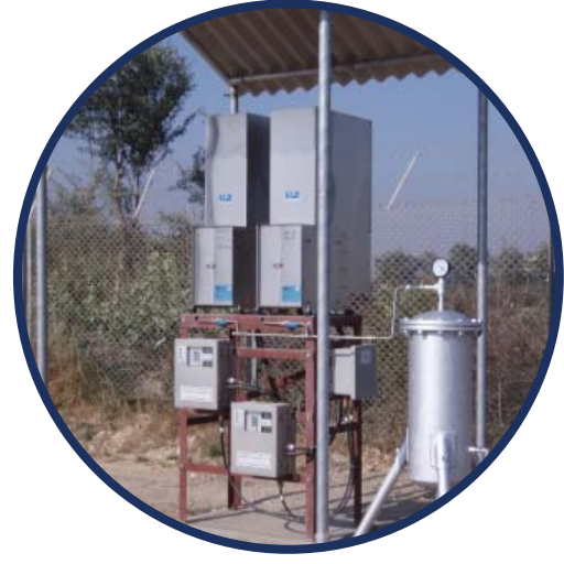
Production: 200 watts for gas well automation and CP - Pakistan
