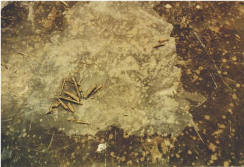
An epoxy coating that blistered was subsequently scraped off, exposing the concrete floor beneath. The surrounding and scattered spots are where blistered caps were removed down to the concrete.
