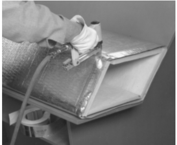
3. Staple flaps on all four sides with 1/2" (13mm) (minimum) outward clinching staples approximately 2" (50mm) on centers.
