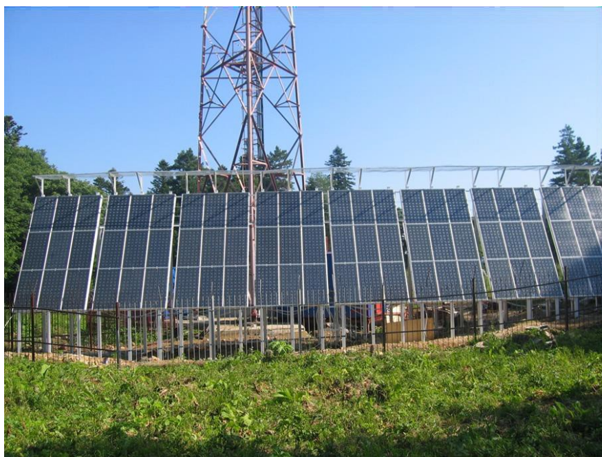
Figure 29 Autonomous 10.8 kW PV system, “MTS” mobile phone station for signal transmission, Lago-Naki, Krasnodar Krai
