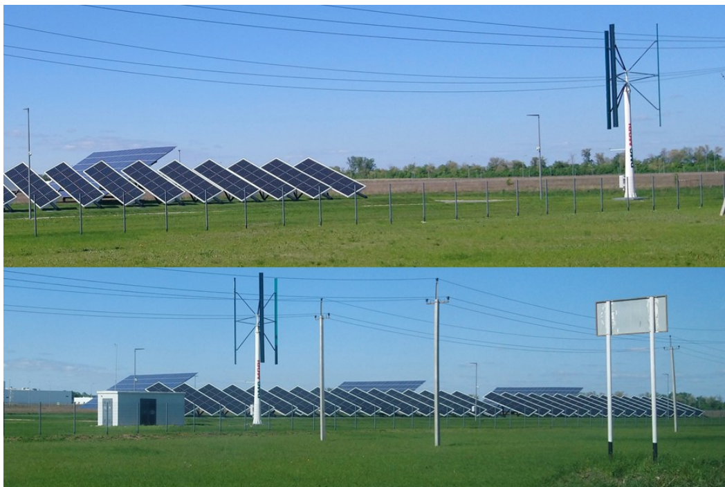
Figure 52 PV system and wind generators at “DGM MORI”, Ulyanovsk
