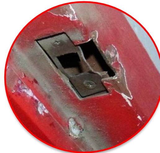
Damaged Strike Plate for Self-Latching Flush Bolt
