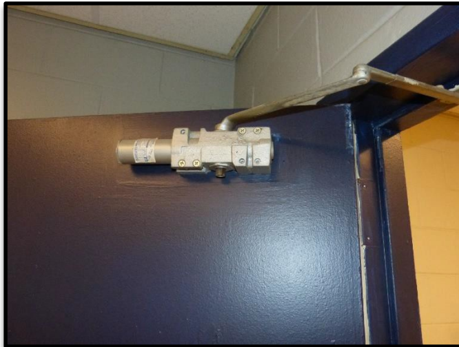
Missing Cover on Door Closer
