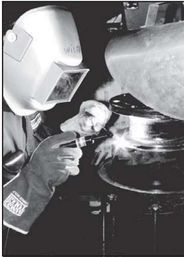
Thorburn's certified welder finishing up the end plate weld on Extra-Flex EFS joint
