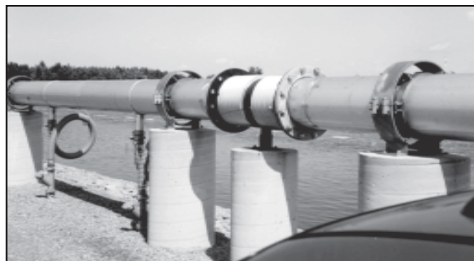
Shown is one of over 20 Thorburn Dual-Flex double expansion joints installed at the Ste-Marthe du Cap-de-la-Madeleine, Quebec, project in 1991
