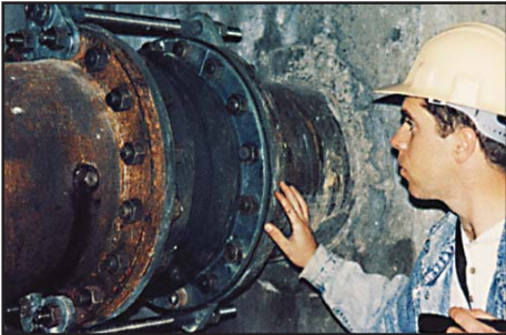
N.B. Power inspecting one of Thorburn's 20 expansion joints at the Belledune New Brunswick Canada power generating station. Size range 1" to 144" I.D.
