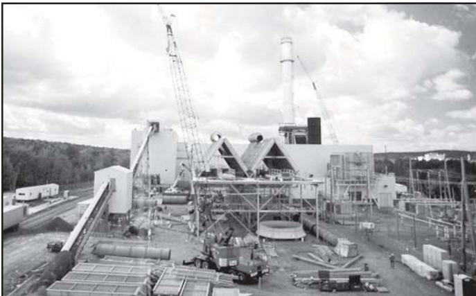
Steam turbine supply lines, condenser and chilled water lines
