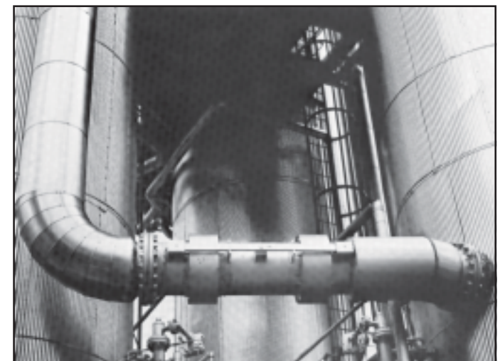
Typical tied universal expansion joint designed for large amounts of lateral movement from the two horizontal lines
