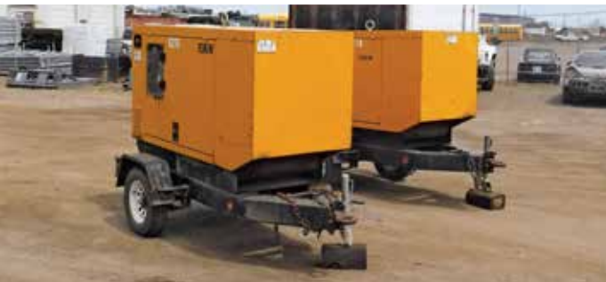
SDMO 30 KW & SDMO 16 KW
