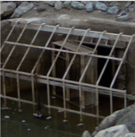
Photo 4 - Side Opening Flap Gate at Nanaimo BC
