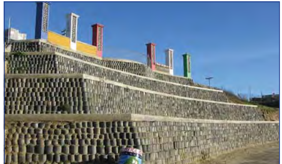
Construction of retaining walls using waste tires may be a way to beneficially reuse waste and reduce sources of trash
