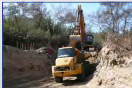
Costly channel clearing operations to remove accumulated sediment and trash and reduce flood risk are needed often in the Valley
