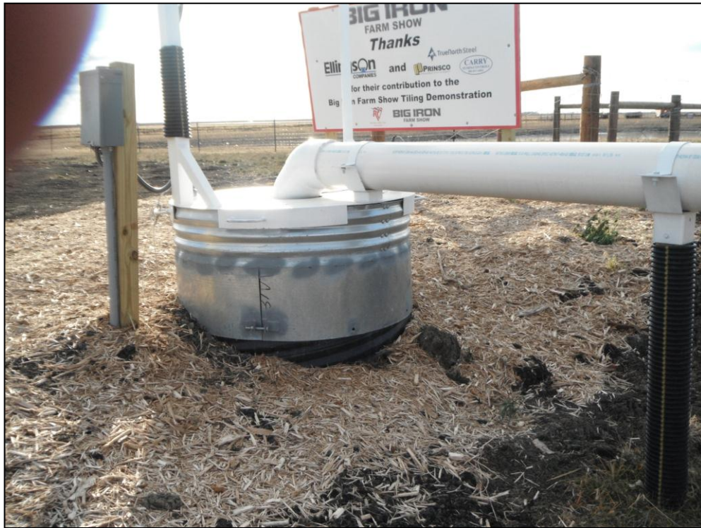
The sump lining is 4 foot diameter corrugated plastic with a metal cover.
