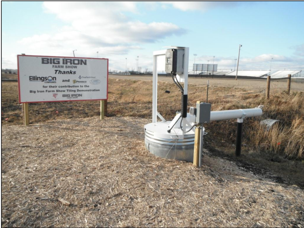
A drainage pump station installed in 2011 in West Fargo, ND. The black box is the VFD controller.
