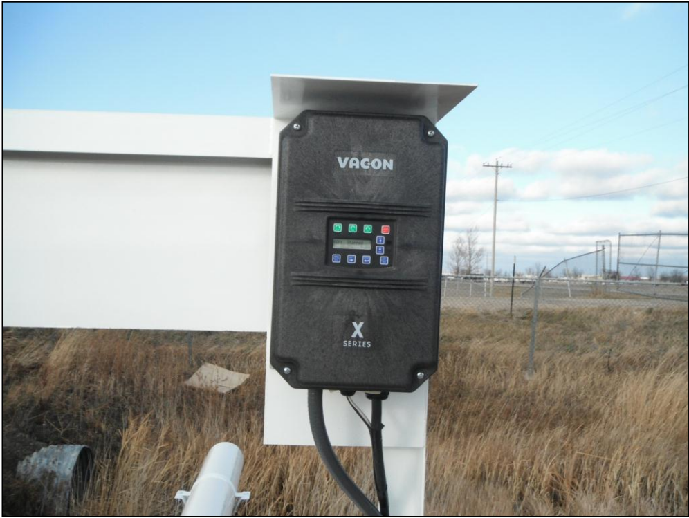
The VFD controller.
