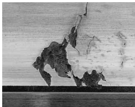
Point Surface Origin (PSO) spalling.
