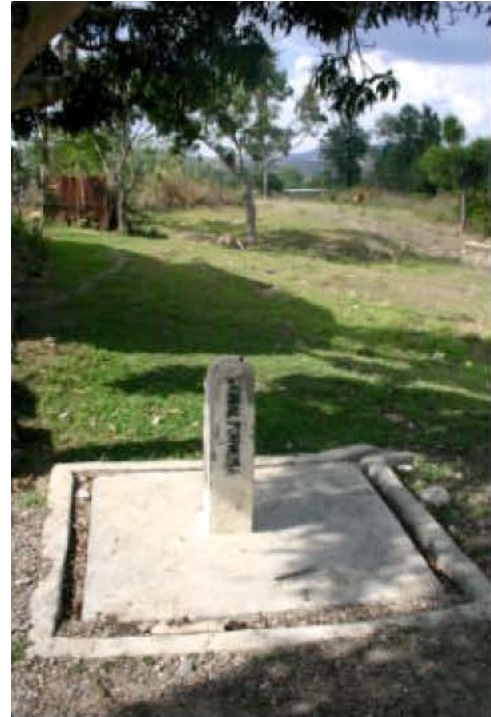
Community-Managed Scheme Vandalized Tap Stand
