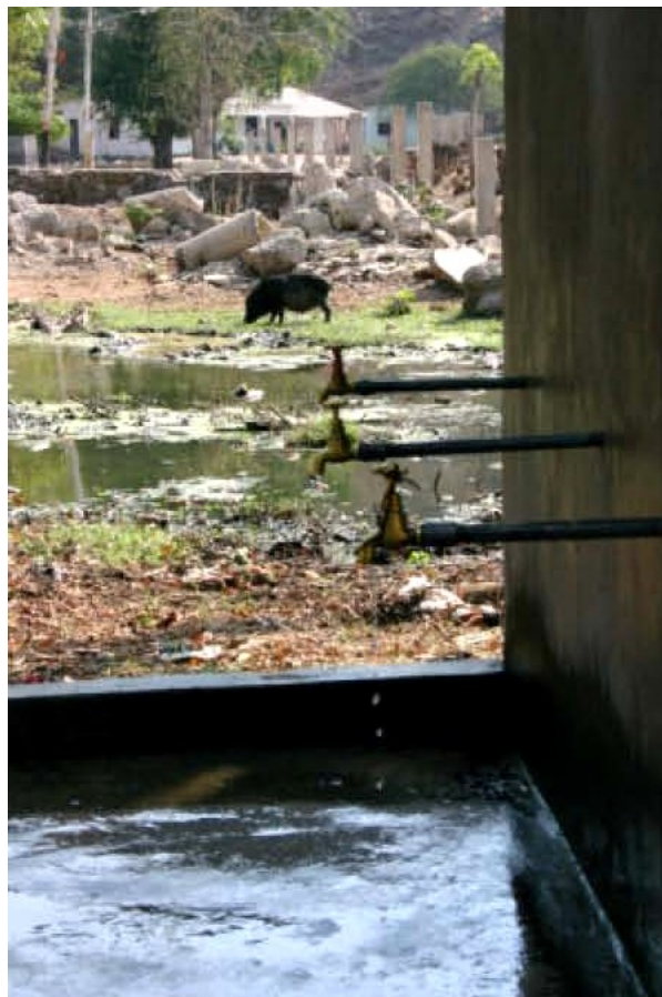
Public Tap Stand in Dili Area Showing Leaking Taps, Poor Drainage, and Animal Presence
