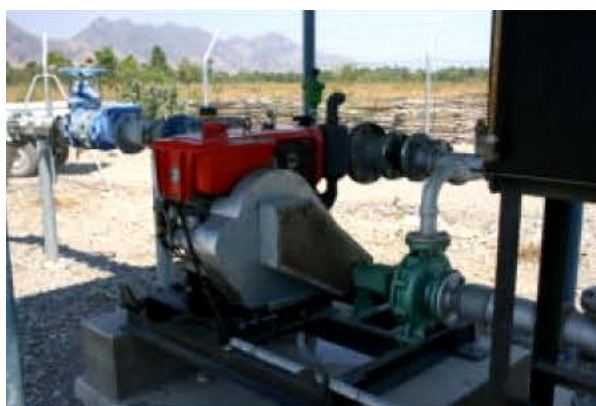
Pump and Motor at Oecussi Bore
