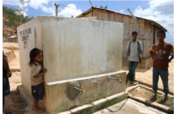
Community-Managed Scheme Missing Taps, Illegal Connection
