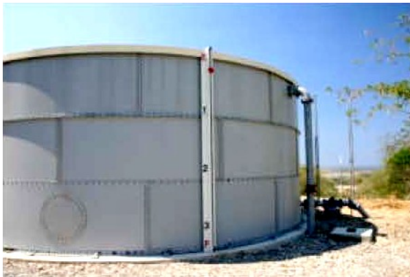
Empty Storage Tank, Oecussi
