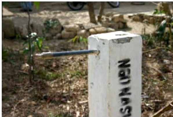
Community-Managed Scheme Missing Tap
