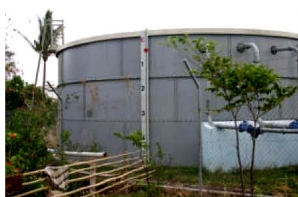
Empty Storage Tank, Maliana
