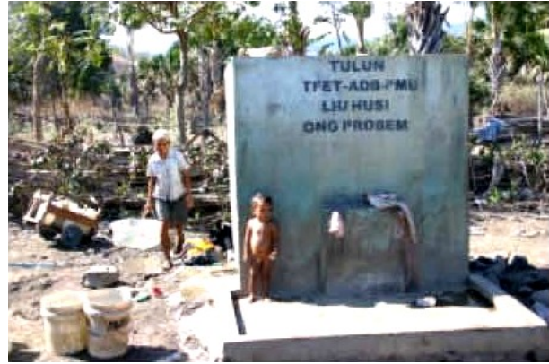
Community-Managed Scheme Non-Functioning Tank and Tap Stand; Pipe Cut to Access Water
