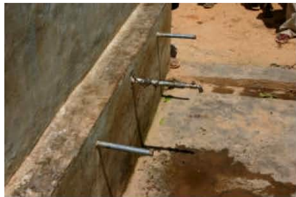
Community-Managed Scheme Missing Taps, No Water
