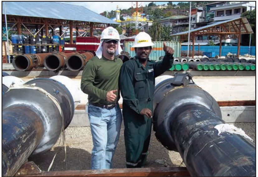
Steve Snyder and coworker Saravana performing ultrasonic testing on butt-joint welds of the low- and high-pressure housing to pipe welds in Fakfak, Indonesia. The temperature was about 110°F that day. The low-pressure housing (typically 30 or 36 in.) provides a location point for the drilling guide base, and provides an interface for the 18¾-in. high-pressure housing. It is important for this first string to be jetted or cemented in place correctly because it is the foundation for the rest of the well.
