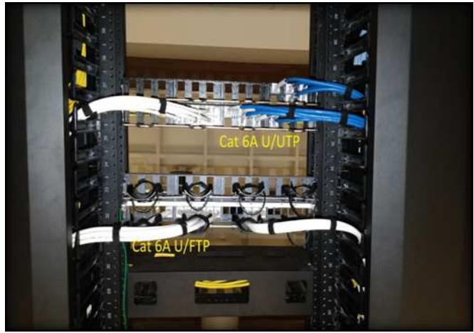
Figure-11: Cables terminated at the Jack Panels
