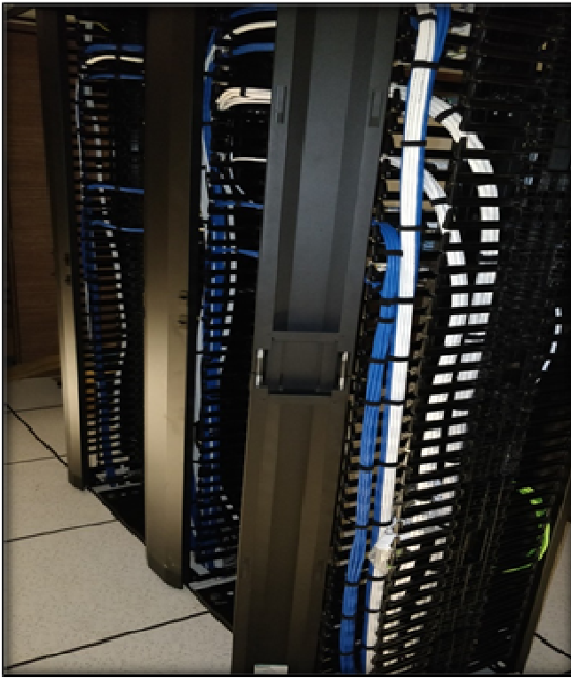
Figure-08: Cables going into the Network Rack
