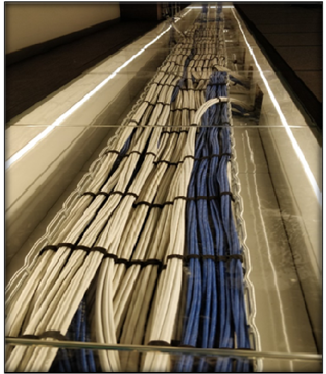
Figure-09: Cables routing in the basket
