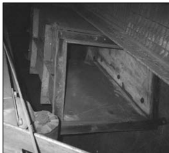
Original rectangular shape transfer chute.
