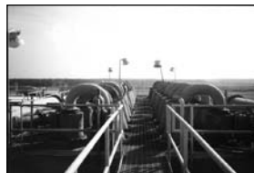
Photo A: 24 hydro-cyclone "overs" discharge lines empty into a 96' long launderer
