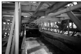
Photo B: The combination of abrasion and corrosion caused by deterioration of the 400 BHN steel used for the launderer
