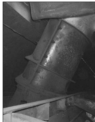
New round steel loading chute is lined with TIVAR® 88.
