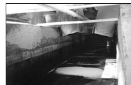
Photo D: After each 24' section was put in place they were field welded into a single 96' long seamless unit. Minimal fasteners (only 24 in the first section) and leading edge protectors complete the installation.
