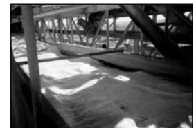
Photo E: TIVAR® 88-2 launderer running full. To date, no signs of wear or corrosion are visible.
