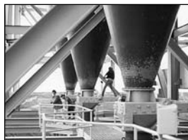
Photo A: Plant personnel would regularly beat on the hoppers when the coal stopped flowing.
