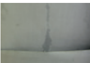
Indoor water damages
