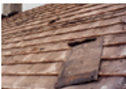
Building structure degradation: mould and mildew.
