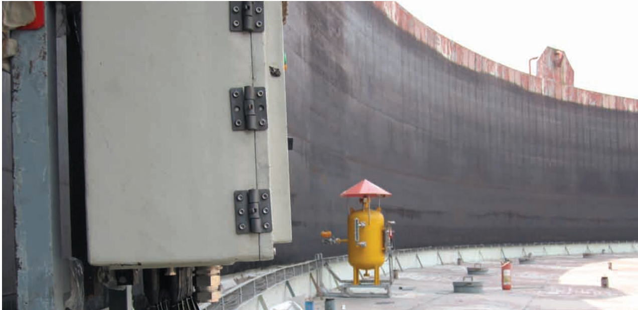
Automatic RIM seal Fire Protection System in Crude Oil Tanks
