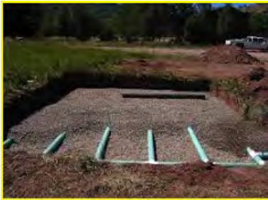
Sand filter underdrains
