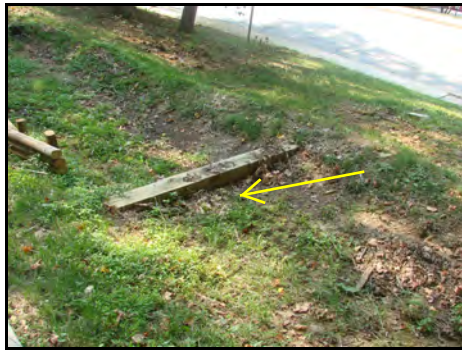
Sediment accumulated behind check dam must be periodically removed
