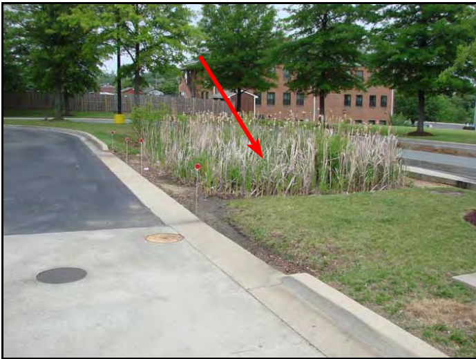
Cattails have taken over this bioretention BMP indicating the surface has been clogged for a long time.
