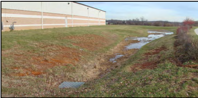
Infiltration basin is failing if water remains on the floor or in trench when 48 hours has passed since runoff ceased entering basin.
