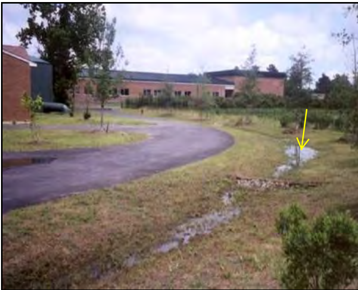
Swale is failing if water does not drain completely within 48 hours after runoff ceases
