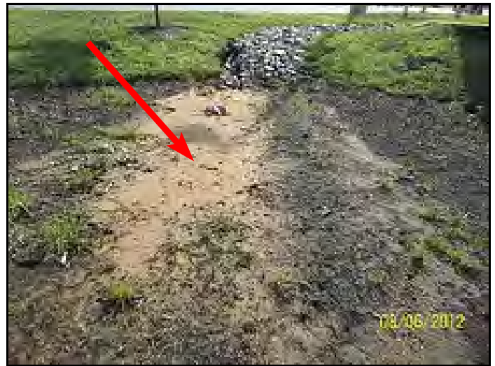
Sediment discharged into bioretention facility from Stormwater Maintenance LLC
