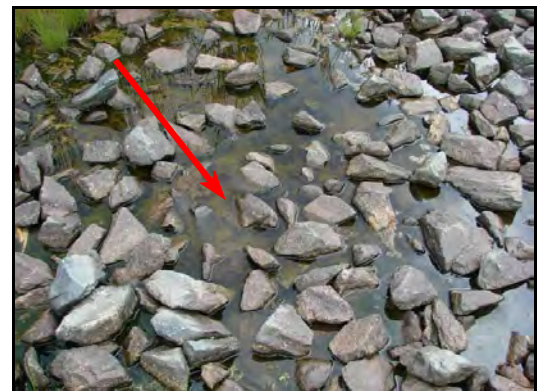
Standing water present in trench more than 48 hours after runoff ended
