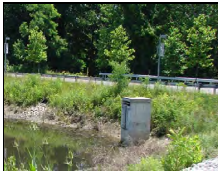
No trees on dam embankment
