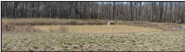
Straight, Level Earth Embankment; No Low Spots; No Trees or Burrows on Embankment
