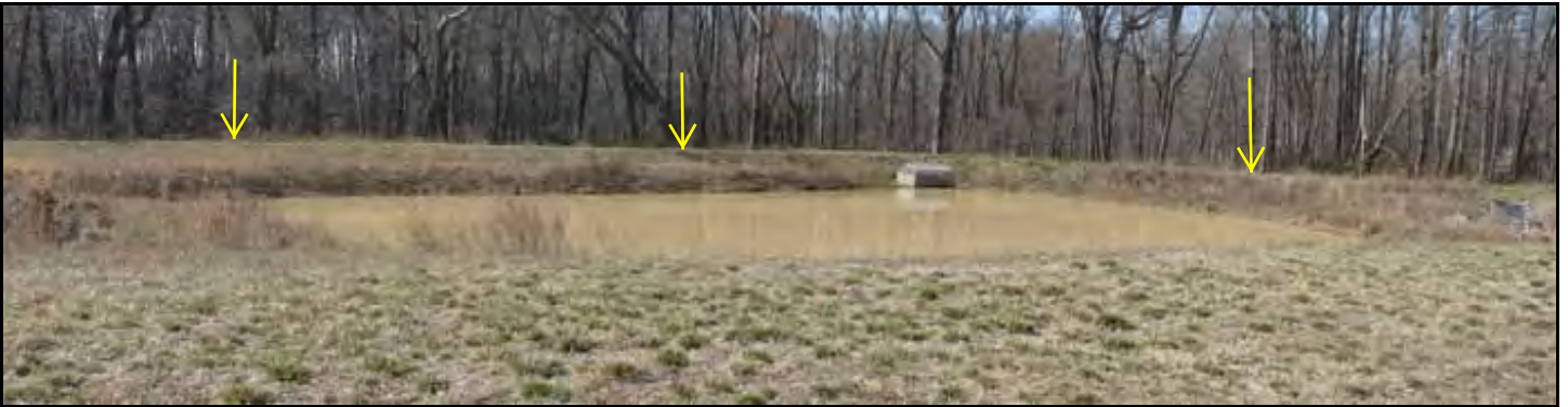
Straight, level earth embankment; No low spots; No trees or burrows on embankment; Arrows point to embankment top, not low-spots
