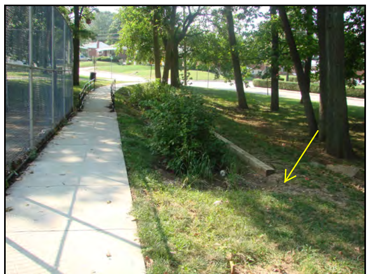
Swale full of sediment; overgrown with vegetation with poor erosion control properties; severe erosion at outlet
