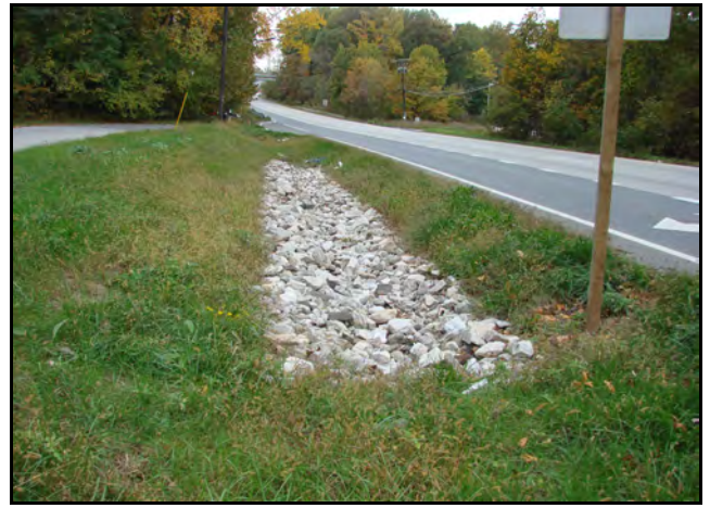
Infiltration Trench (IT) Stone or gravel usually exposed at surface often with observation well
