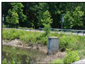
No trees on dam embankment
