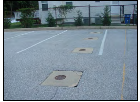
Infiltration Trench beneath parking lot; only well/cleanout covers visible; can't be assessed
