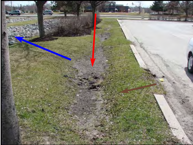
Sediment from parking lot (right) captured in forebay (center) to protect infiltration trenches (left)
