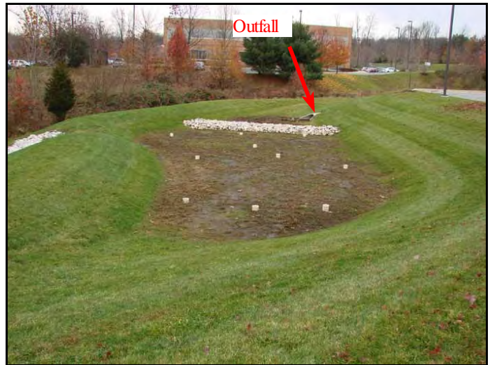
Sand Filter with PVC clean-outs; checkdam forebay to capture sediment discharged from storm drain outfall in upper right
