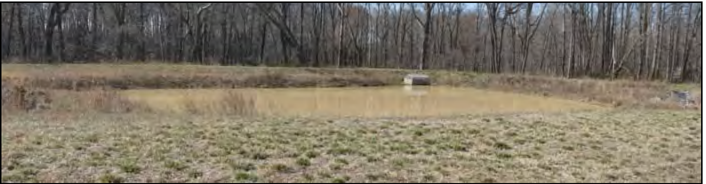
Straight, Level Earth Embankment; No Low Spots; No Trees or Burrows on Embankment
