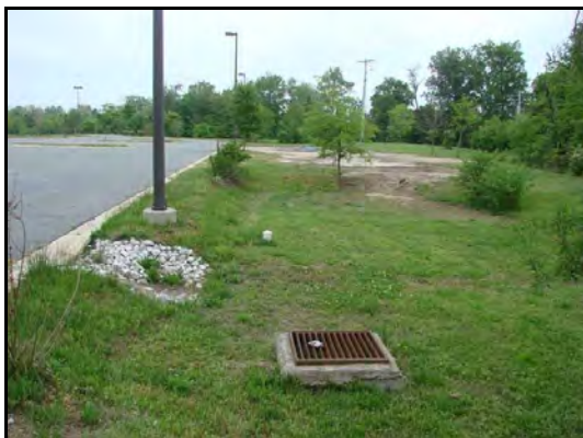
Exposed soil, like that above this bioretention BMP, can quickly kill an infiltration trench
