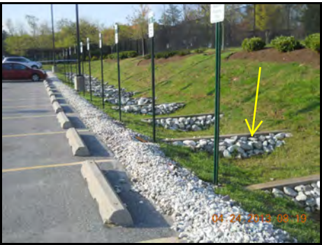
Some swales, particularly those with steeper slope, have stone, wood or concrete check dams to enhance infiltration
