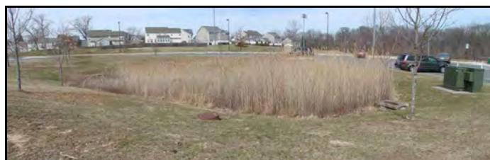
Same overgrown sand filter as it looks in winter
