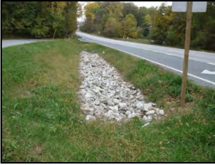
Infiltration Trench with exposed stone; most common type
