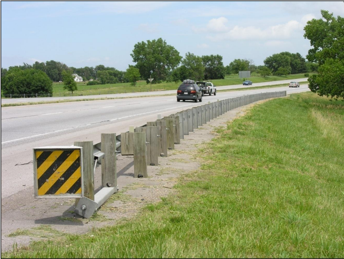
Figure 21. Upstream side guardrail end-terminal
