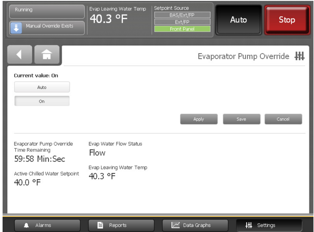
Figure 25. Manual Control Settings screen (Evaporator Pump Override shown)
