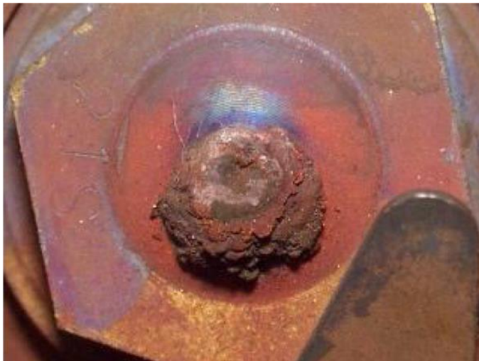
▲ Figure 25. Leached copper from tracing lines can fall out of solution during condensate flashing and block a trap's orifice.
