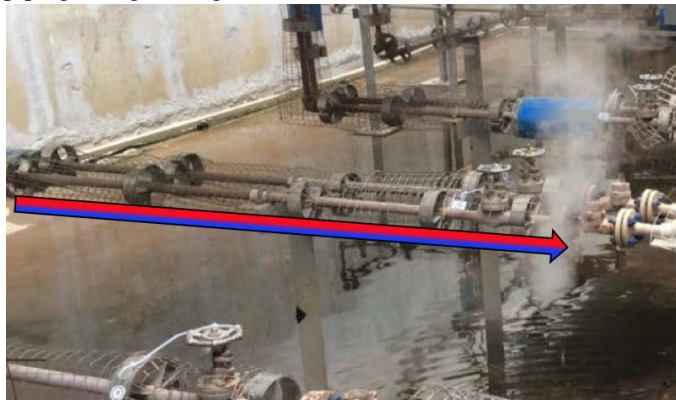
▲ Figure 22. Long horizontal piping runs to the traps created steam locking issues, needing internal bypass models to resolve.
