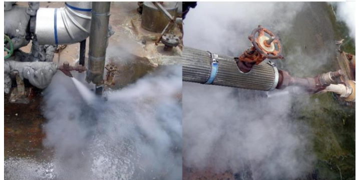
▲ Figure 2. Opened bleeds are a sign of poor heat transfer.
