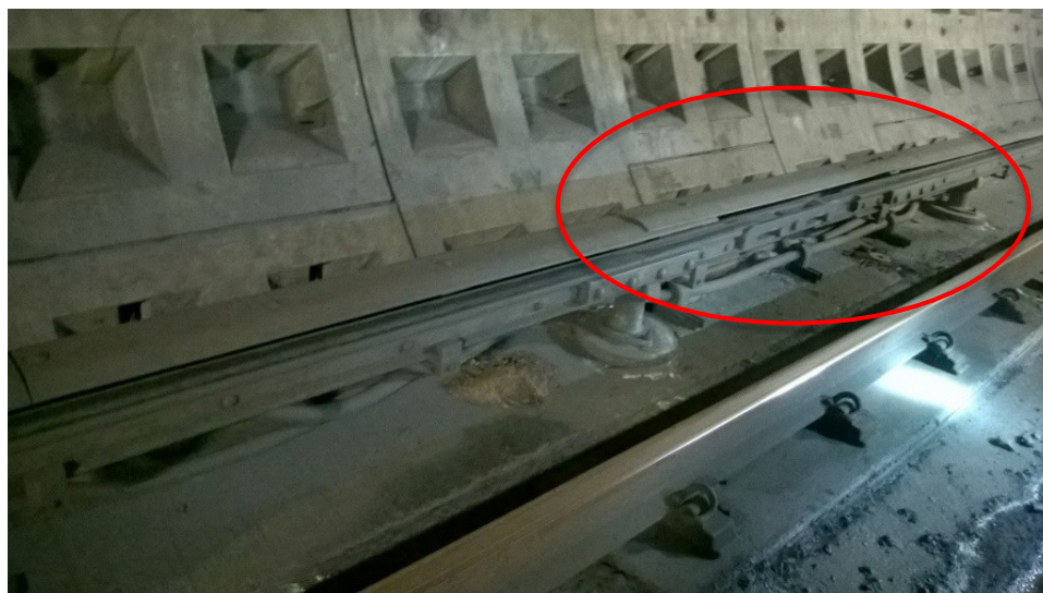
Figure 7: Third Rail Expansion Joint and Jumper Cables
