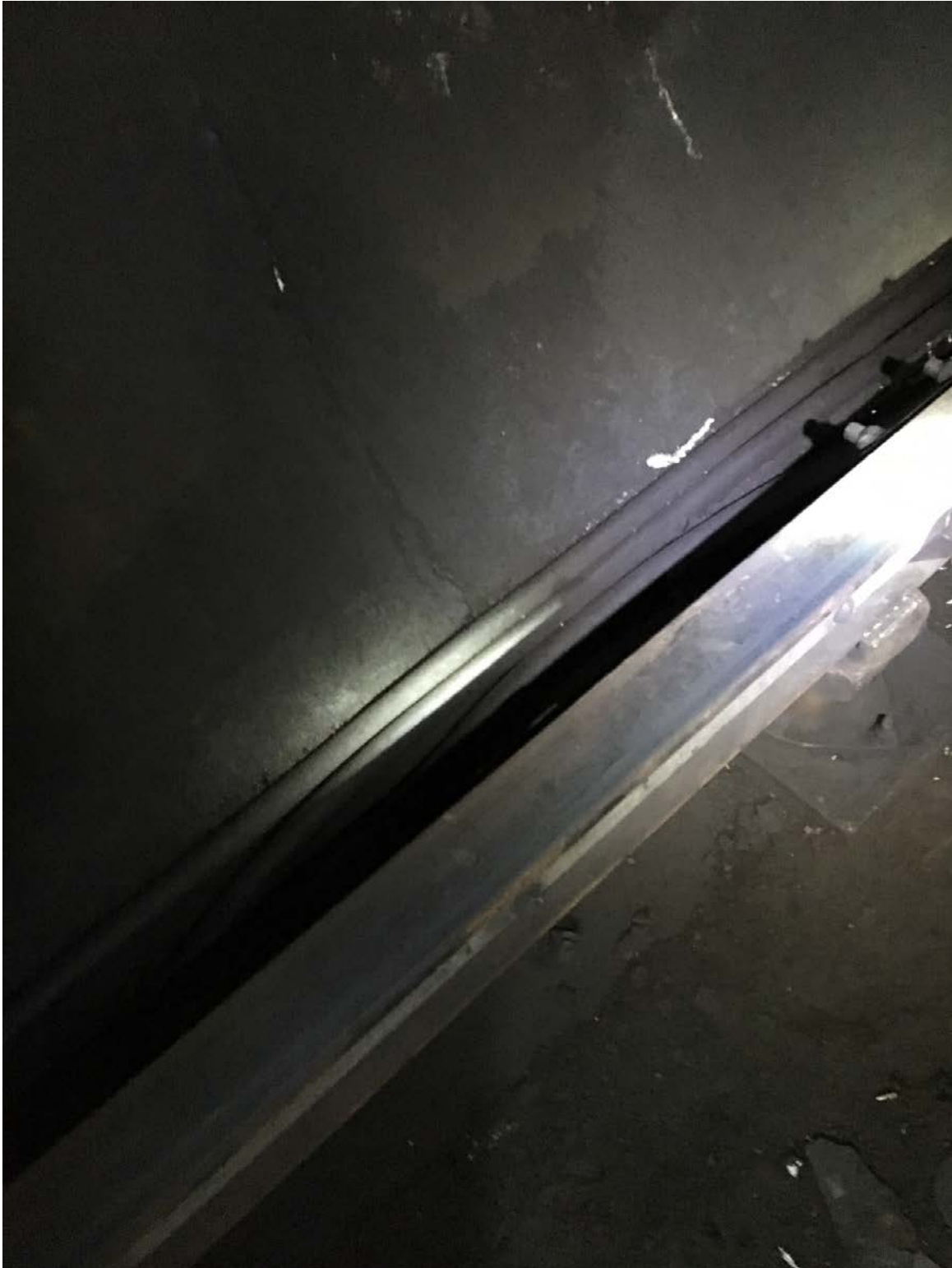
Figure 15: Power Cables Loose against Tunnel Wall
