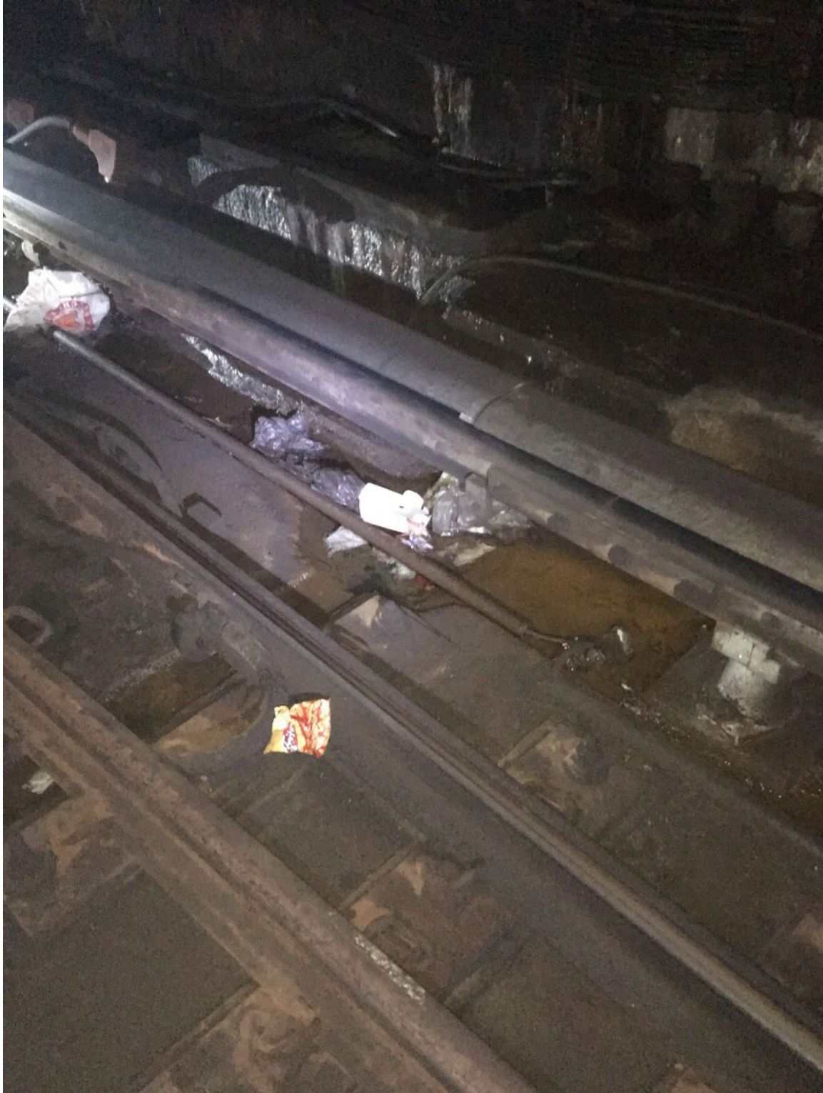
Figure 11: Water and Debris under Third Rail
