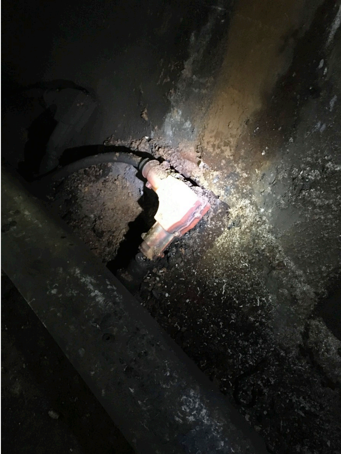
Figure 10: Cable and Connector Assembly Coated in Mud and Water
