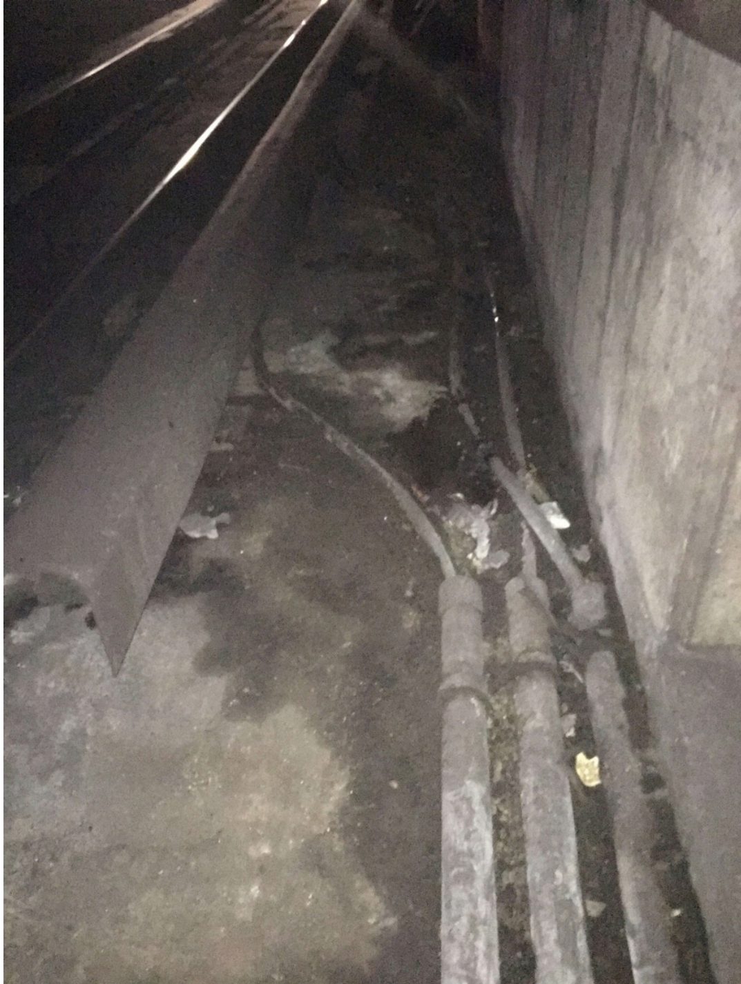
Figure 12: Power Cables on Tunnel Floor in Damp and Muddy Conditions
