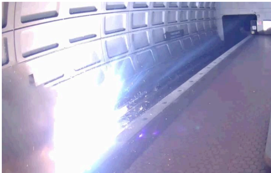
Figure 2: Electrical Arcing Event at Federal Center SW Station on May 5, 2016
