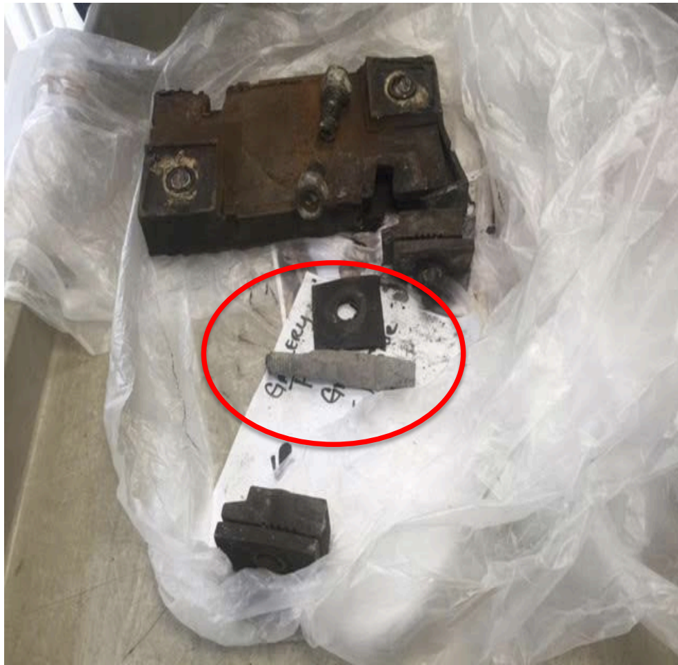
Figure 16: Track Fastener Involved in Gallery Place Electrical Arcing Incident, June 27, 2016
