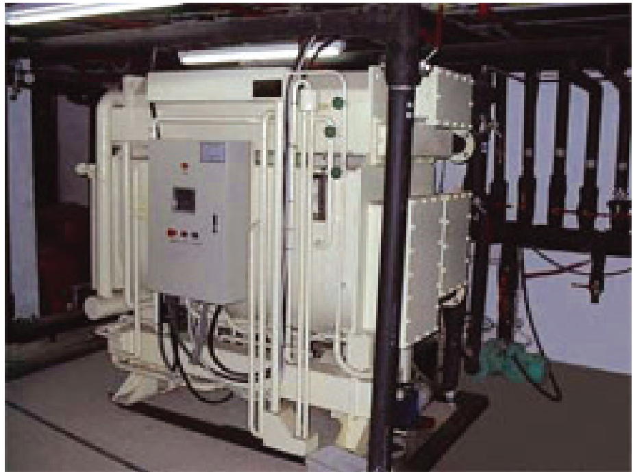
Fig. 4 Absorption chiller – Rethimno village hotel - Crete
