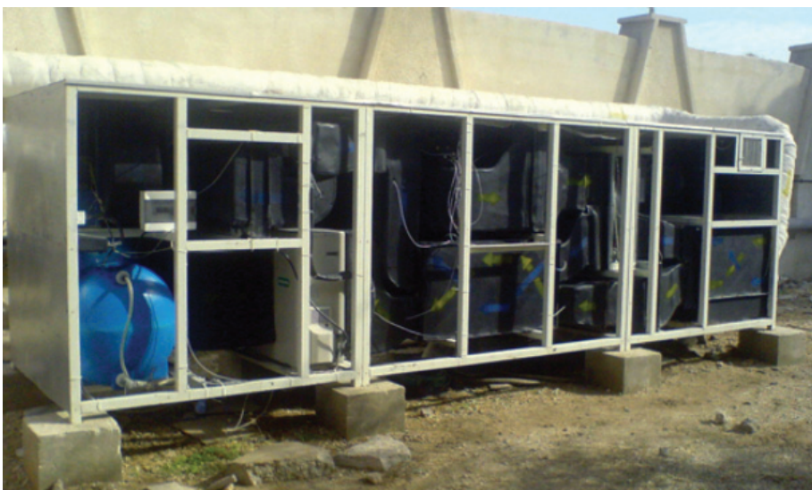
Fig. 6 The installed solid desiccant air conditioning unit in Kish Island
