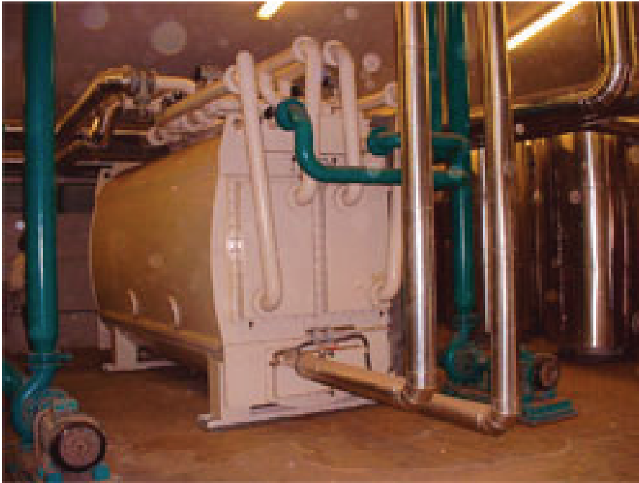
Fig. 5 Adsorption chiller - Sarantis - Greece
