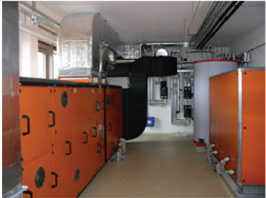
Fig. 7 Liquid desiccant cooling system, installed at the new "Solar Building Innovation Center (SOBIC)" at Freiburg (D).
