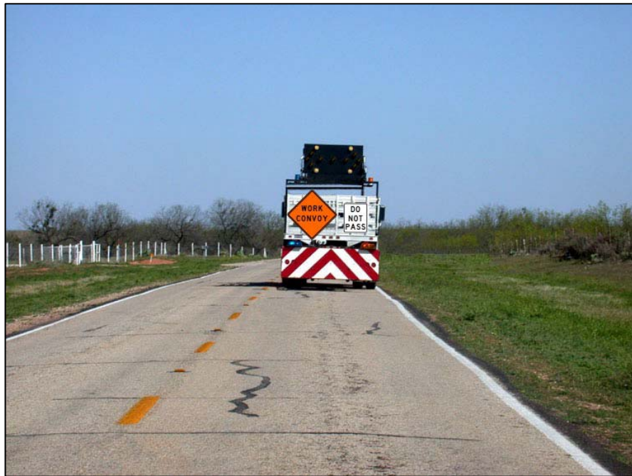
Figure 16. Addition of a DO NOT PASS (R4-1) Sign.
