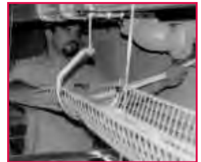
CatTrax installed at the BICSI Headquarters Expansion
