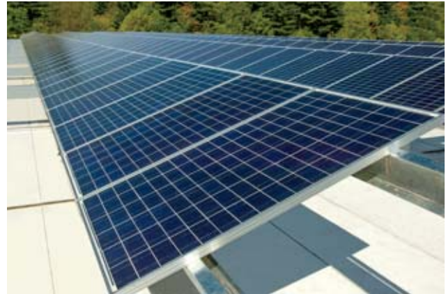
Andover, Massachusetts solar project
