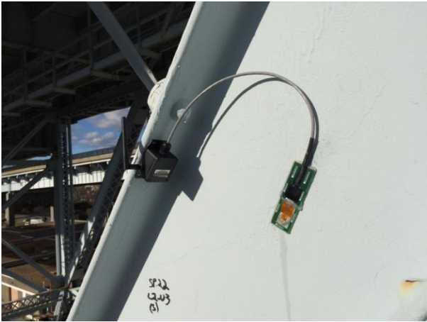
Figure 1: Resensys strain SenSpot sensor installed on a steel truss chord
