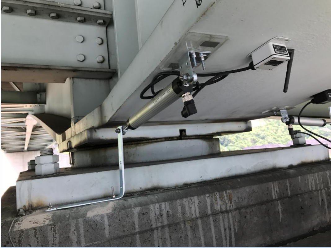
Figure 5: Displacement SenSpot sensors to monitor an expansion joint
