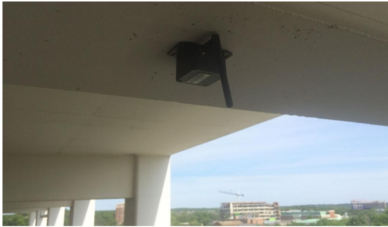
Figure 7: Acceleration SenSpot sensor installed on a bridge in Indonesia
