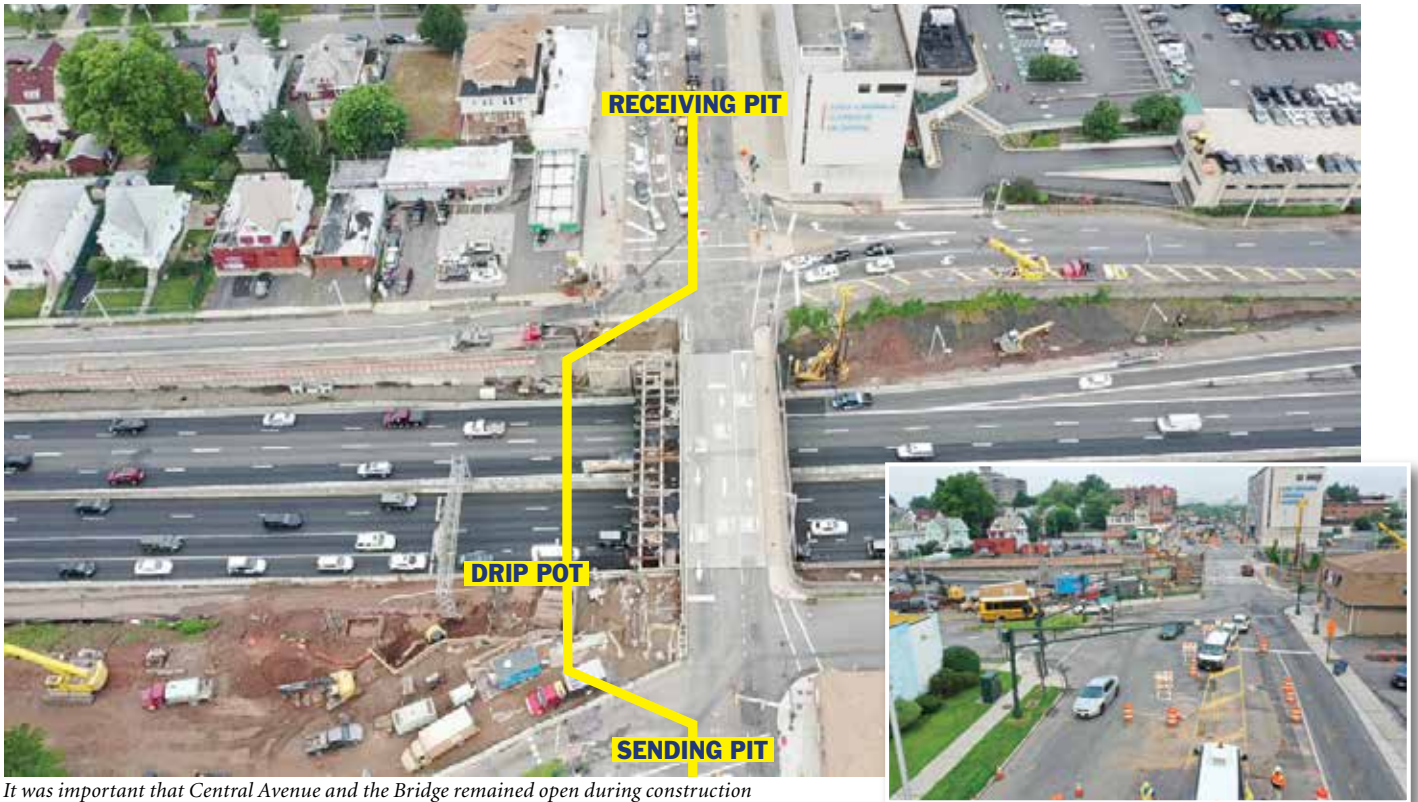
It was important that Central Avenue and the Bridge remained open during construction
