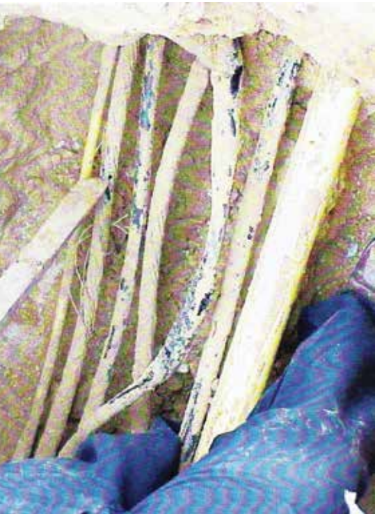
Precise location of conflicting buried lines is critical
