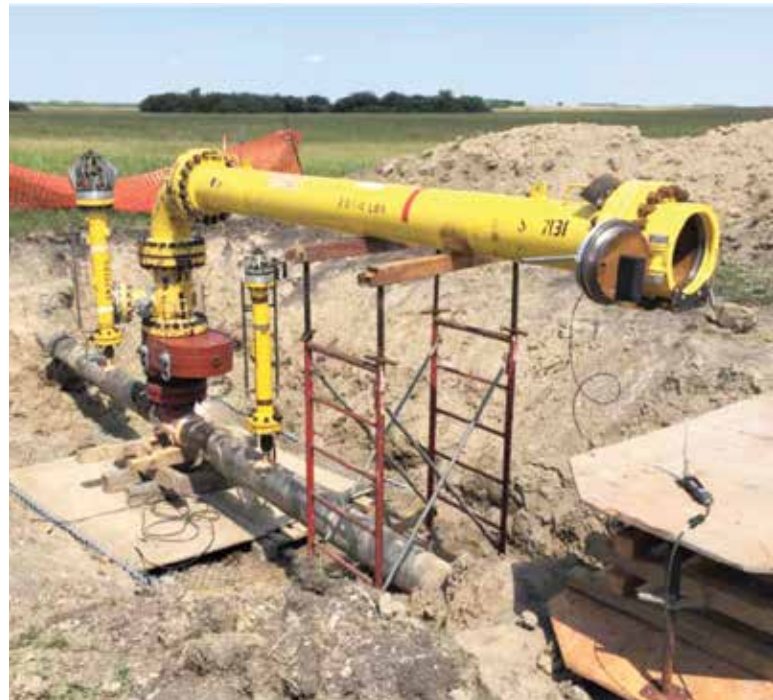
Figure 6: Pipetel's Launch System for Explorer 10/14
