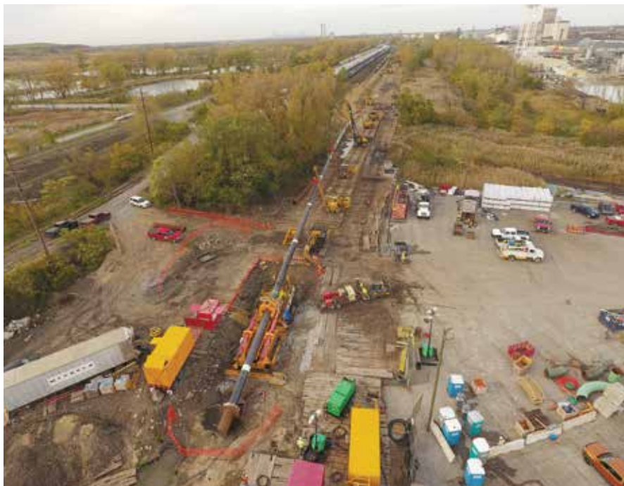
Extensive right of way was required as staging area for the pipe
