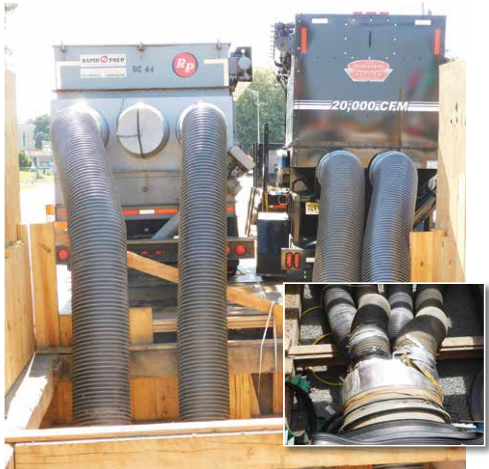
Maintaining a minimum 45mph velocity was an achievement, considering pipe diameter and geometry
