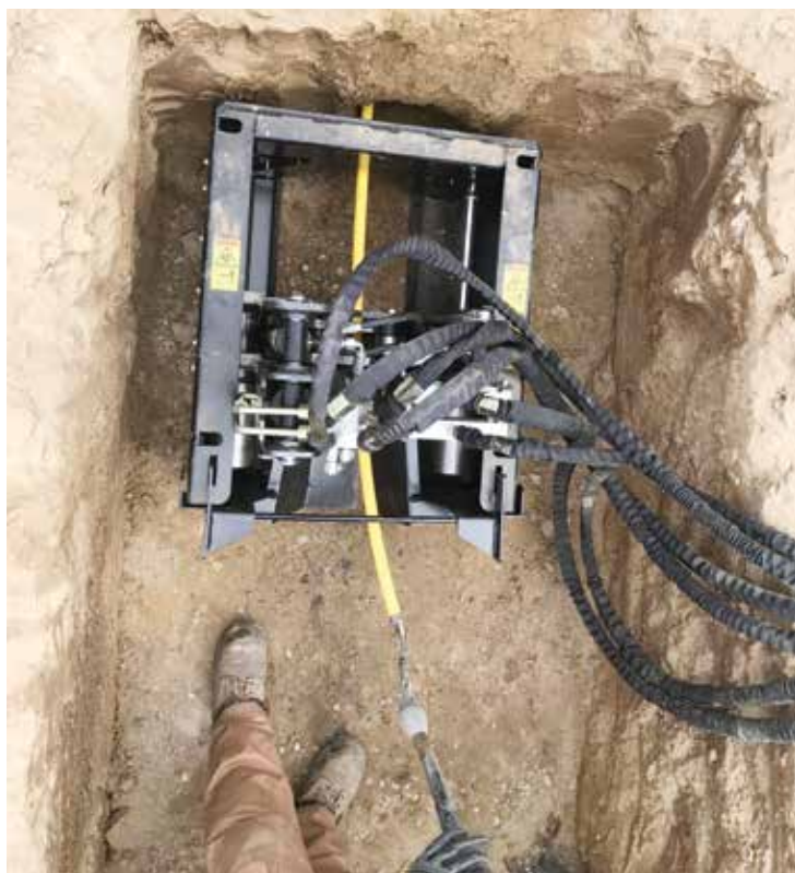
PE product pipe is pulled into place simultaneously as the existing pipe is extracted
