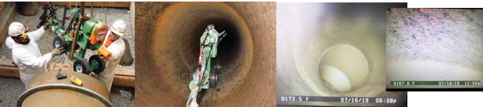
Self-propelled robotic sand blast unit, “The Beast” efficiently cleaned the metal to a NACE-2 finish
