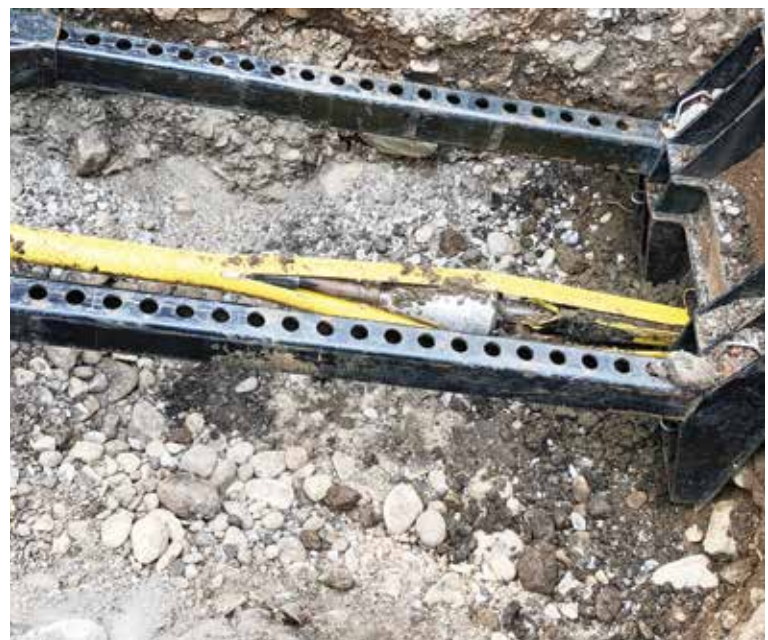
Trenchless pipe slitting is a proven method for replacement of plastic pipes that utilizes the same location as the existing line
