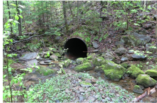
Figure 1. Buried corrugated metal pipe under a highway used as a stream crossing.
