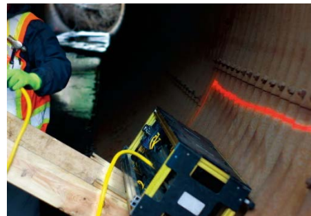
Figure 7. Shows the BCT hardware being deployed in a CMP structure.
