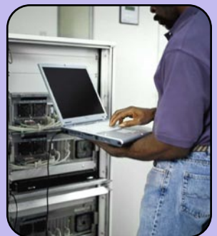
Calibration within the power cabinet.
