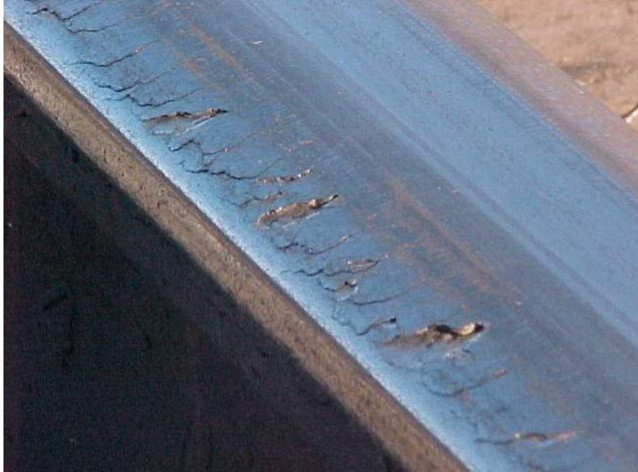
Figure 51: Gauge Side Head Checking and Flaking
