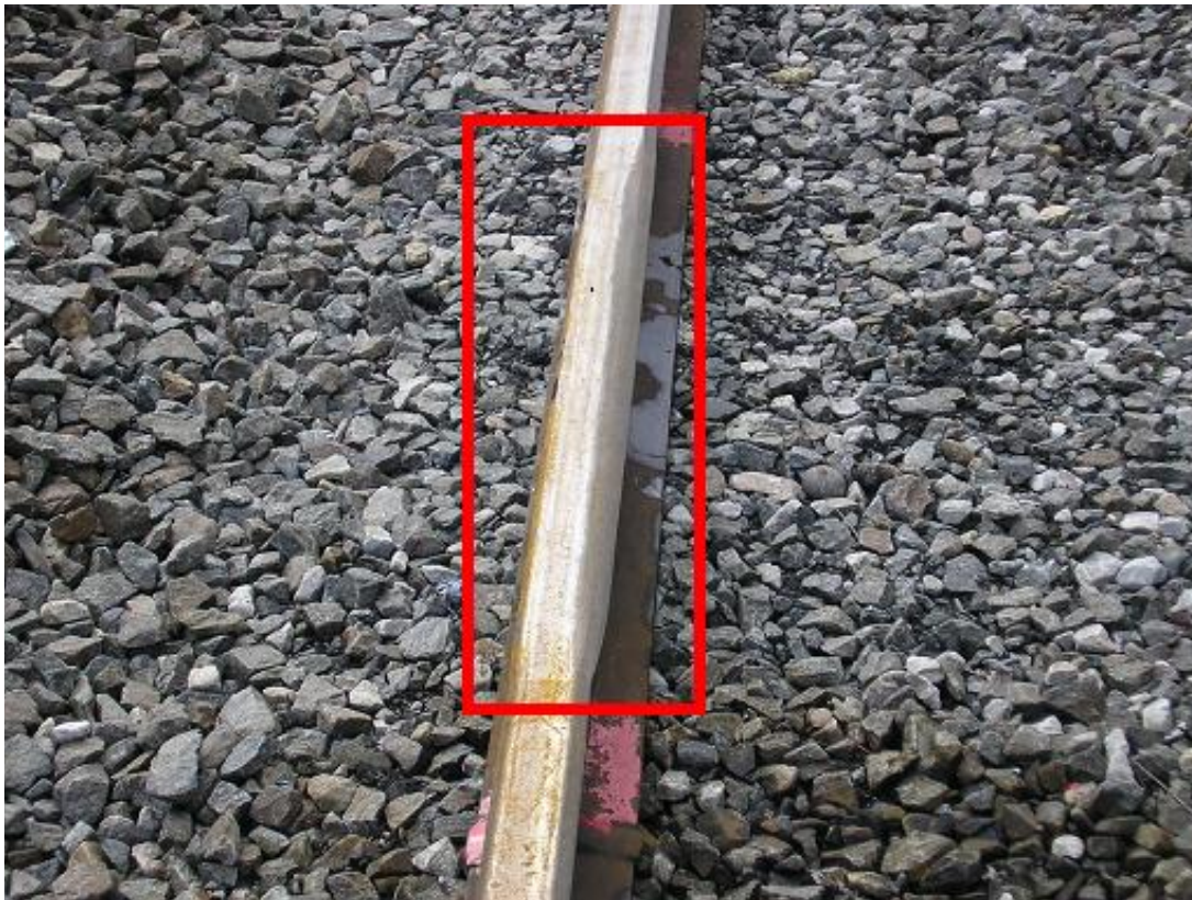
Figure 27: Shear Break Showing Dark Discoloration Identifying Defect Length
