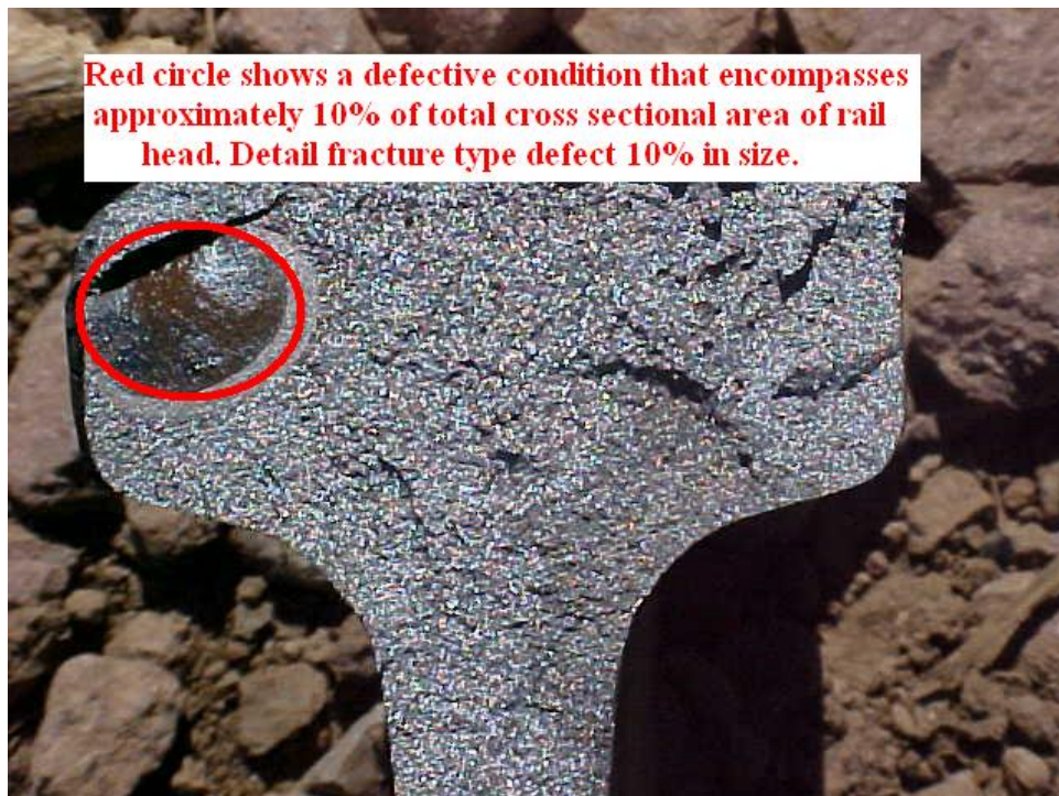
Figure 1: Identifying Transverse Defects in Relation to Cross Sectional Area of Rail Head
