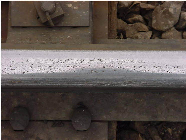
Figure 49: Centralized Flaking Condition Showing Chipping of Parent Metal
