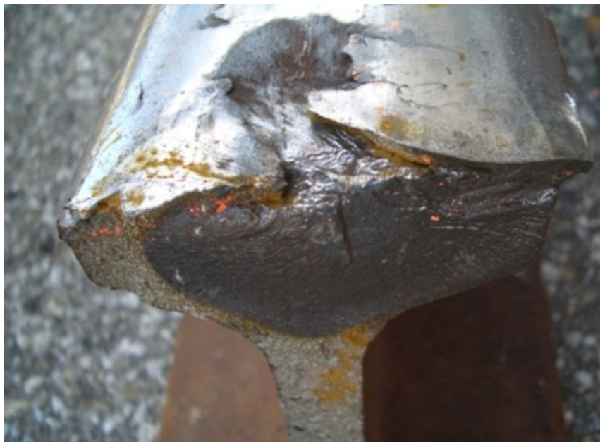
Figure 20: Engine Burn Fracture Showing Significant Growth
