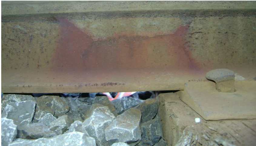
Figure 30: Split Web Defect Showing Bleeding Condition Along Crack Development
