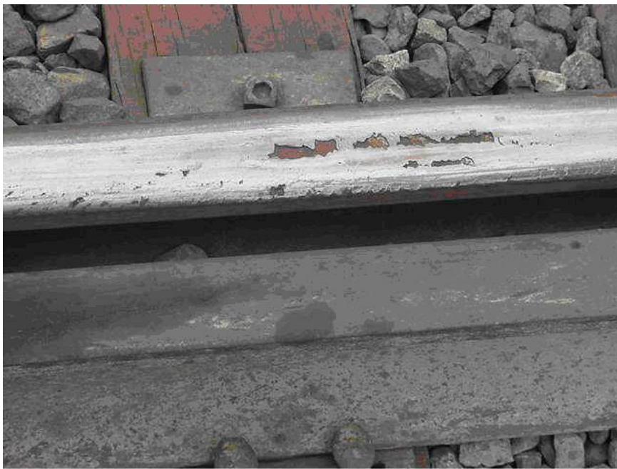
Figure 52: Flattened Rail Head Showing Displacement of Parent Metal (Spalling)
