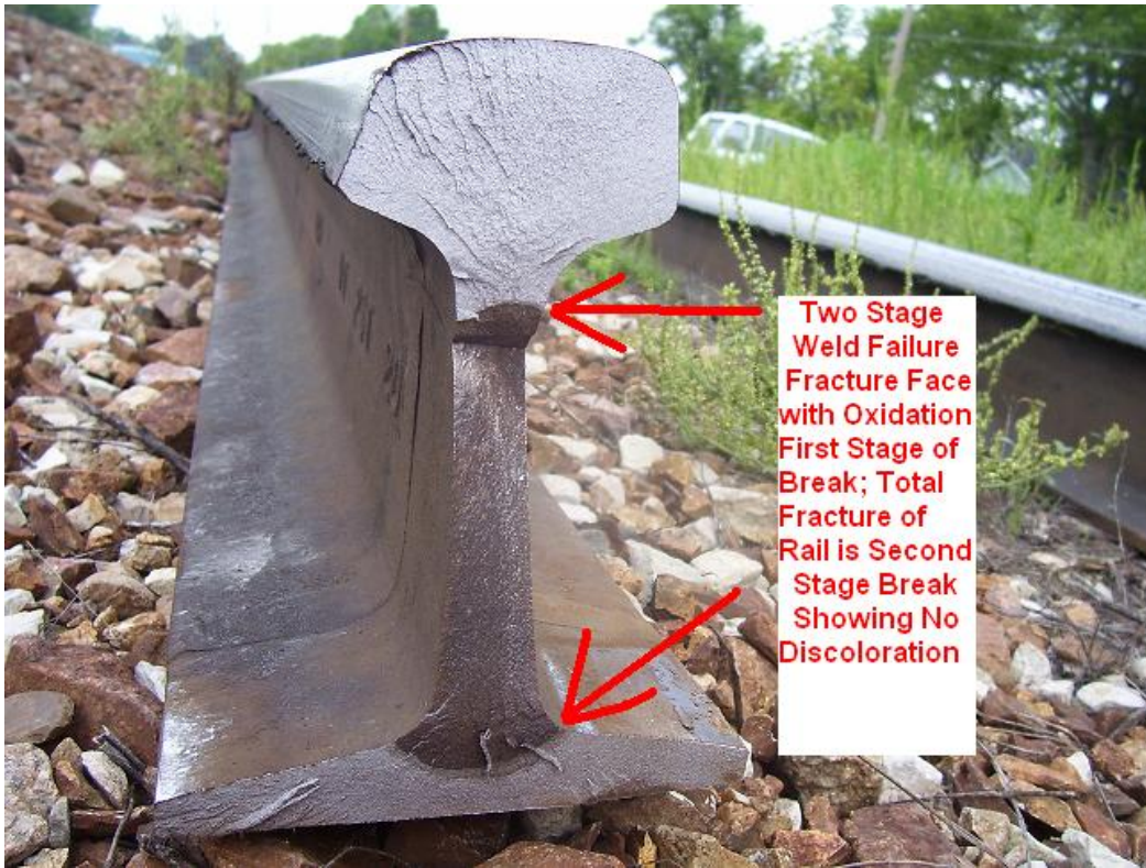
Figure 9: Weld Failure Showing First Stage Fatigue Development and Second Stage Rupture
