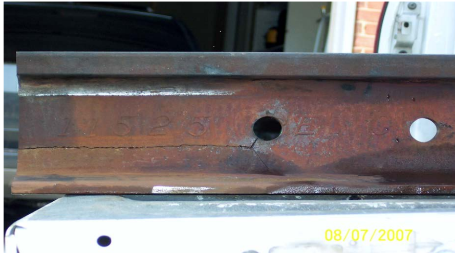
Figure 43: Bolt Hole Crack Originating in Lower Quadrant with Significant Progression
