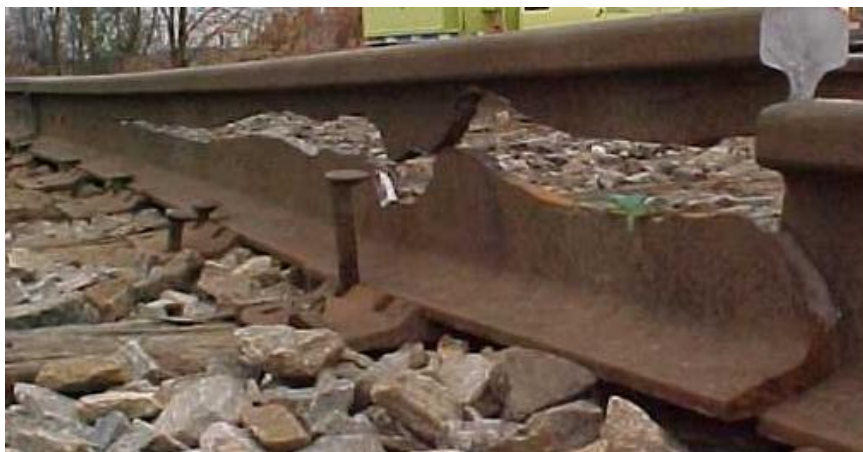
Figure 31: Web Failure Resulting from High Residual Stress
