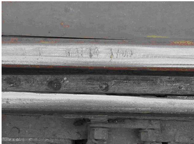
Figure 50 Thermal Cracks on Burned Stock Rail
