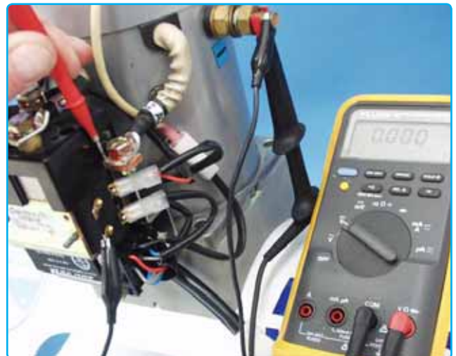
Checking voltage on A2 with ground to blue jumper attached
