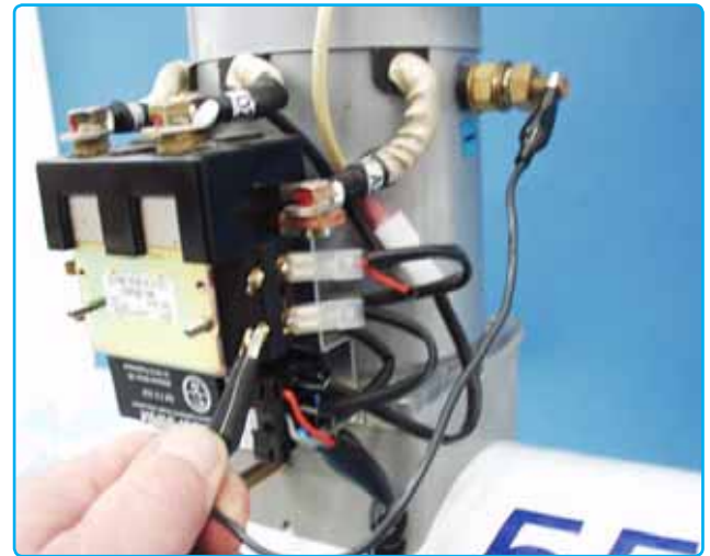
Jumping ground to blue on D2 coil
